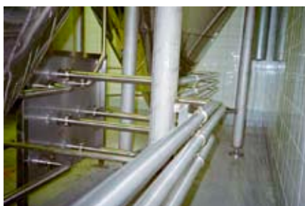
Backside of a two tank panel in the tankhouse at Fruängskällan
