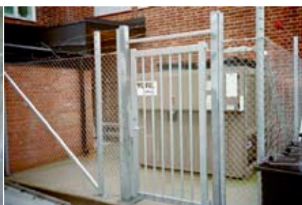
Outside installation of York cooling equipment at Fruängskällan
