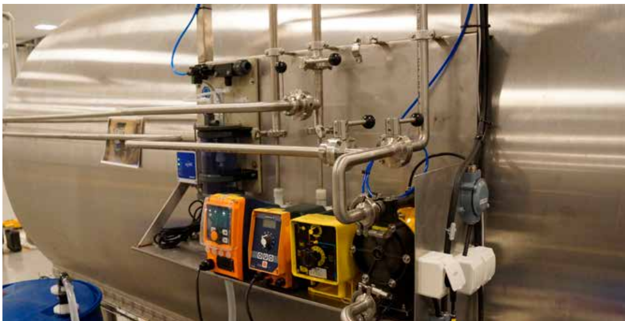
Dosing pumps CIP Wellnox
